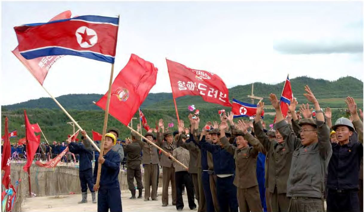
Young builders successfully finish the concrete tamping of the dam of Paektusan Hero Youth Power Station No. 1 in August 2015.
